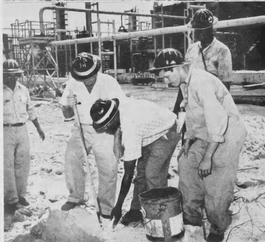
AT THE site of the dismantled No. 12 aviation unit, Mechanical-Yard employees recently had the job of blasting out concrete foundations. A double-rope blasting mat, top photo, confines debris. Workmen, above, charge a hole with several sticks of dynamite.
